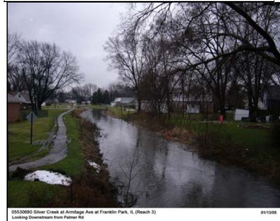
05530680 Silver Creek at Armitage Ave at Franklin Park, IL (Reach 3) 01/13/08 Looking Downstream from Palmer Rd
