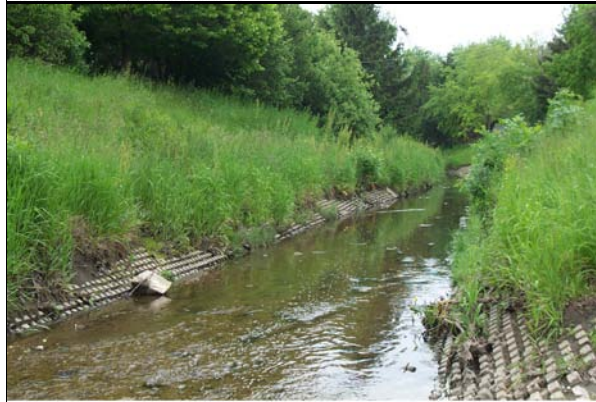
05529990 Weller Creek at William St at Mt Prospect, IL (Reach 2) Looking Downstream from School St 06/03/03
