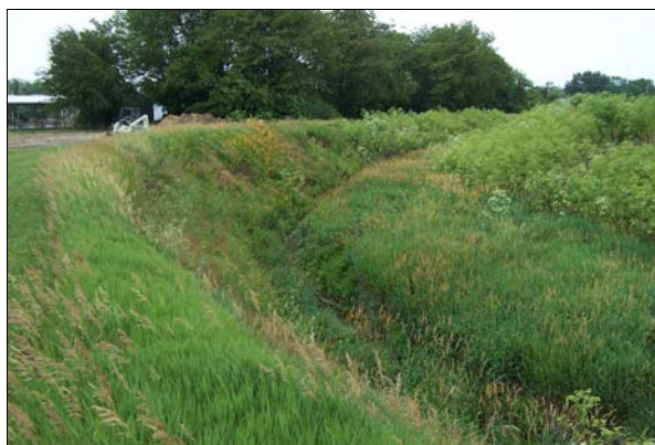
03343800 Kickapoo Creek at Mattoon, IL Looking Upstream, overgrown grass at bend 06/15/04
