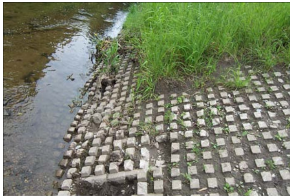
05529990 Weller Creek at William St at Mt Prospect, IL (Reach 2) Closeup of cement biostructure at School St 06/03/03
