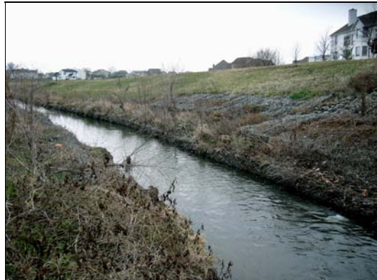
05590060 Copper Slough at Staley Rd at Champaign, IL Looking downstream, below Staley Road 04/28/06
