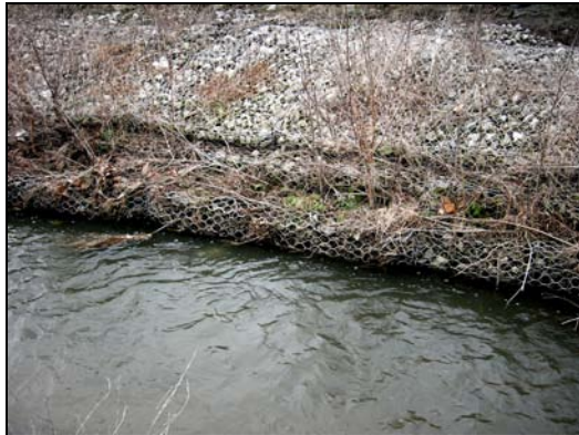
05590060 Copper Slough at Staley Rd at Champaign, IL Gabion boxes, west of Staley Rd. 04/28/06
