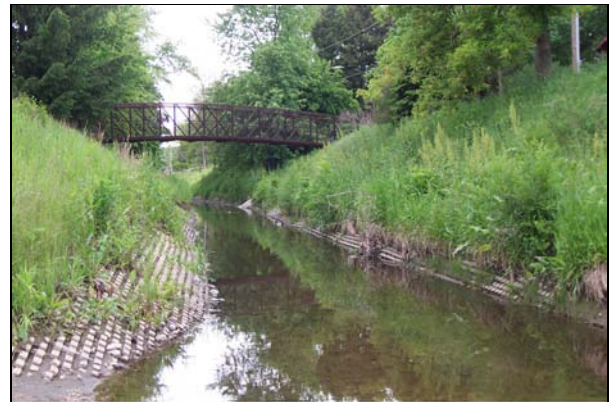
05529990 Weller Creek at William St at Mt Prospect, IL (Reach 2) Looking Upstream at cement bank protection (at School St) 06/03/03
