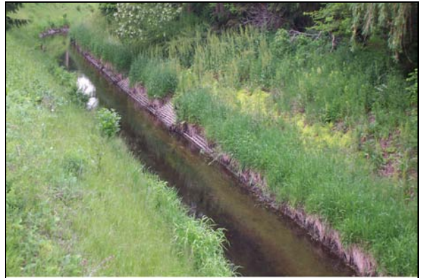
05529990 Weller Creek at William St at Mt Prospect, IL (Reach 2) 06/03/03 Looking Upstream of Williams, cement
