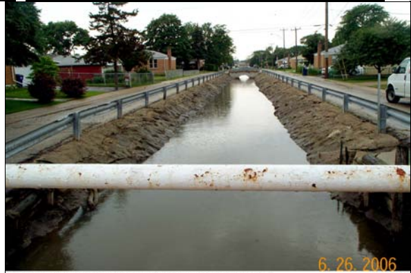
05530670 Silver Creek at Scott Ave at Franklin Park, IL (Reach 5) 06/28/06 Looking upstream
