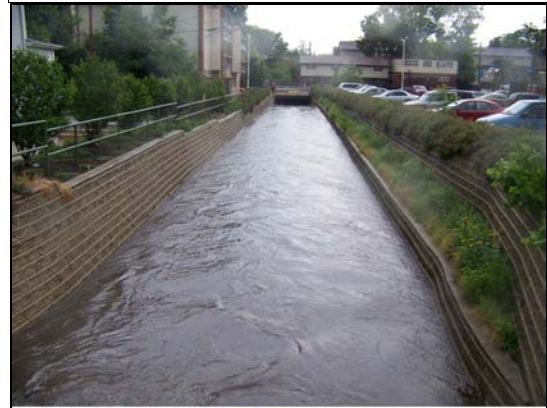
03337100 Boneyard Creek at Lincoln at Urbana, IL Looking Downstream from Gregory St
