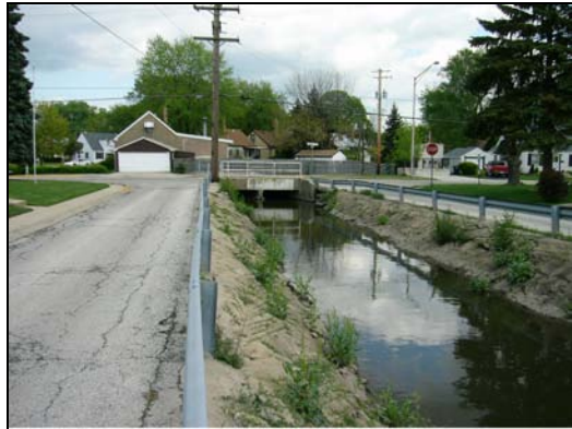
05530670 Silver Creek at Scott Ave at Franklin Park, IL (Reach 5) 05/02/06 From Louis St, looking downstream
